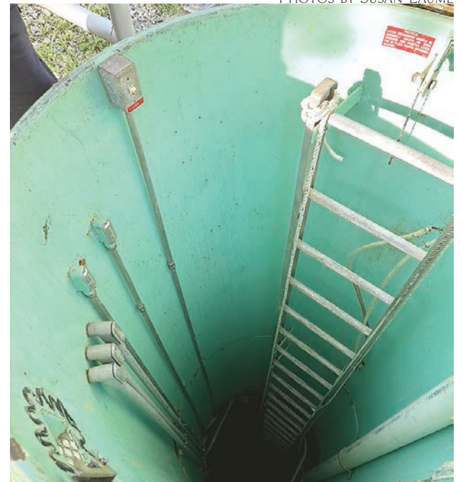
Deep below, sewage under pressure is flowing to the station's tank to be pumped to the next high point, so gravity can assist the movement toward the treatment plant
