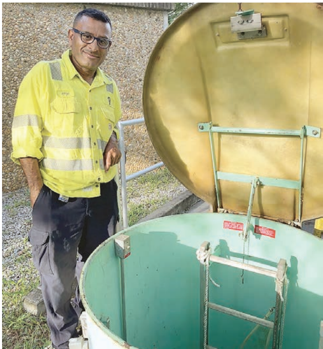
Fifteen year employee Jorge Maldonado, of Fairfax, stands at a wet-well access pipe while completing a weekly inspection of the Workhouse Road pumping station.
