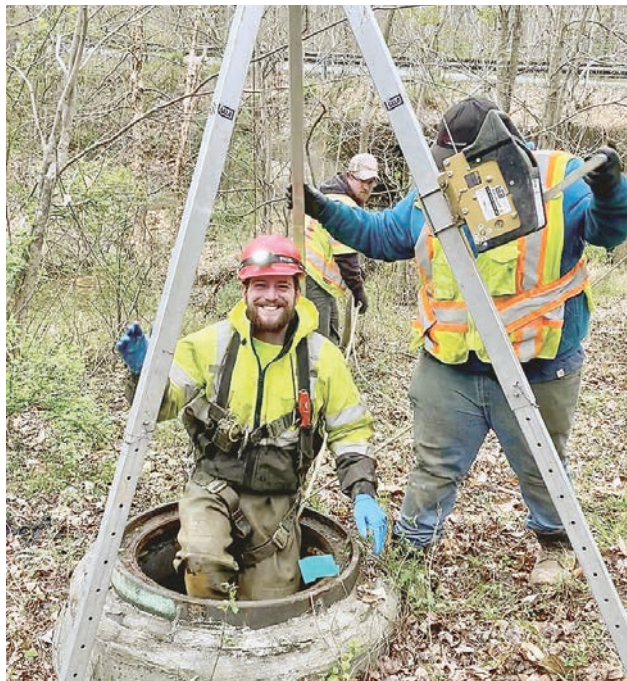
Hundreds of miles of sewer pipes are inspected annually with cameras, sensors, and lasers to assess pipe condition, sometimes requiring entry into the system to retrieve entangled equipment
